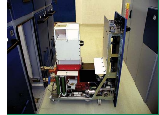
Carriage with high-speed circuit breaker
