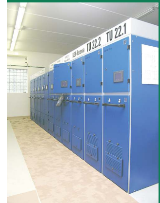
Cabinet configuration of traction power supply technology
